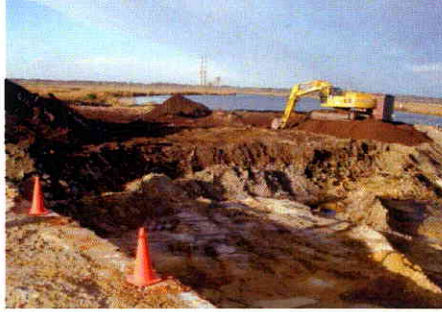
Excavation and off-site disposal of approximately 107,000 tons of soil and sediment with visible (magenta) slag or magenta staining
