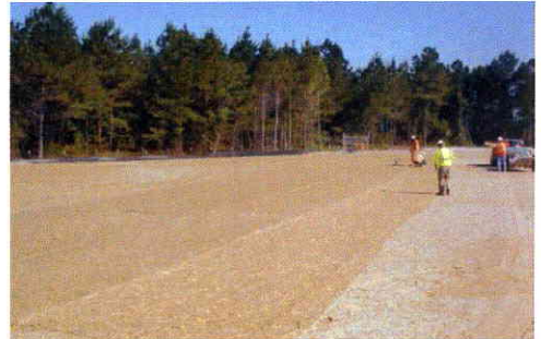
Installation of 1-foot thick soil covers over areas of residual lead and arsenic containing soils, and seeding
