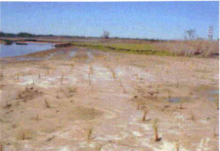
Backfilling of the marsh excavation area with imported clean fill and vegetation with native marsh plants
