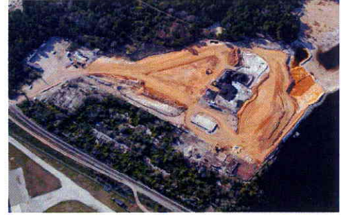
Backfilling of the upland area excavation with imported clean fill, and seeding
