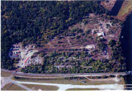
Site clearing and demolition of select structures. Approximately 1,200 tons of demolition debris were disposed of off-site
